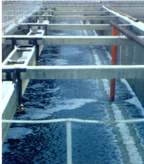
Fig. 3.4. Aeration tank with pneumatic aeration system
